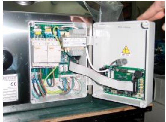
control box inside
